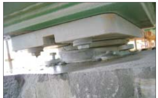
Bearing incorrectly installed. Over rotation due to poor grout bed. Fasteners not tightened. Additional washers used as packers. Void between top plate and super structure. Stainless steel sliding surface painted on site.
