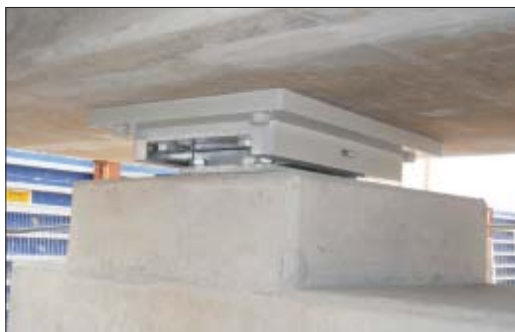
Mechanical guide bearing and upper adaptor plate correctly installed. All bearing interfacing surfaces are horizontal. All surfaces are free from contaminants.
